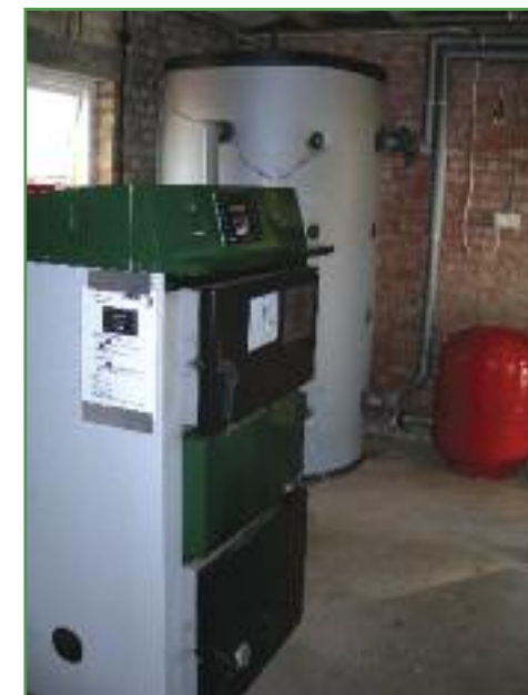
A modern high-tech woodfuel heating system for a local four bedroom house.
